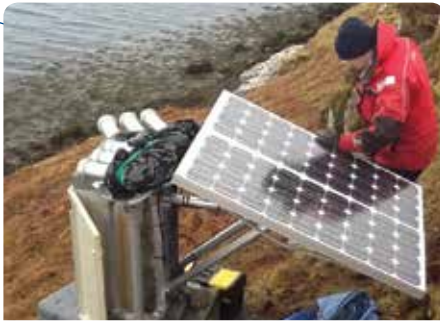
solar powered sector lights
