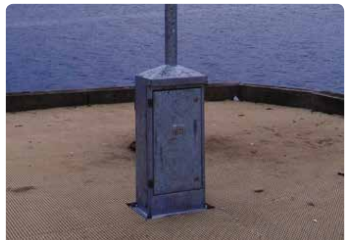
mains power operation
